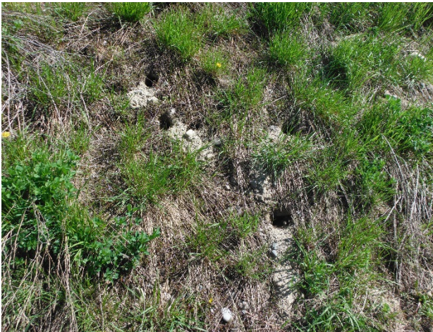
5.05: May 10, 2017 Rodent Burrows at Toe of West Gypsum Dike
