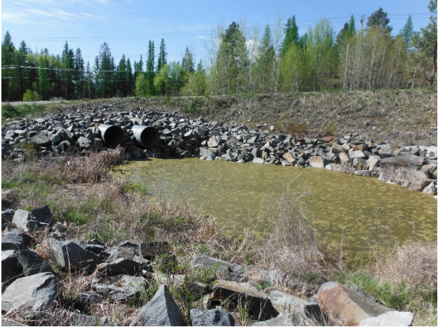
9.07: May 10, 2017 Ponded water in stilling basin at end of ESP Emergency Spillway
