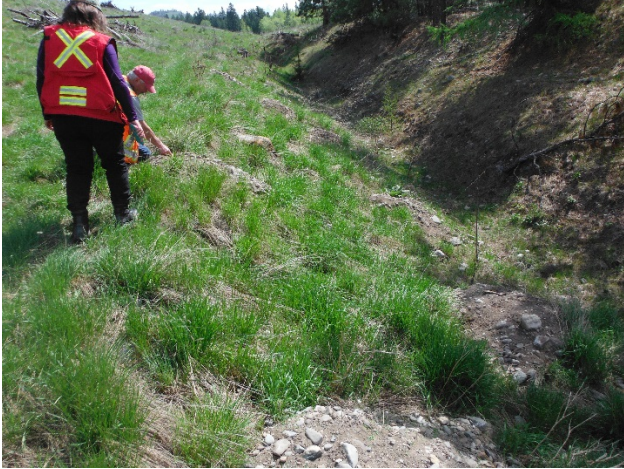
5.19: May 10, 2017 Rodent burrows upstream of ditch at dike toe
