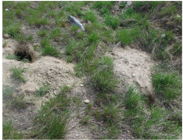
5.22: May 10, 2017 Rodent burrows in ditch at toe
