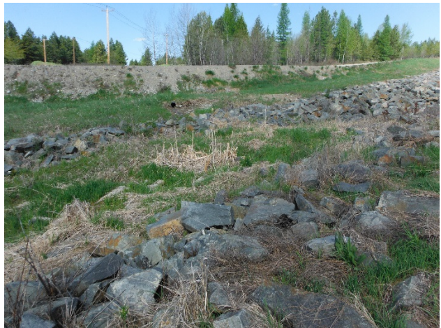
9.06: May 10, 2017 Vegetation growing in Spillway channel near base
