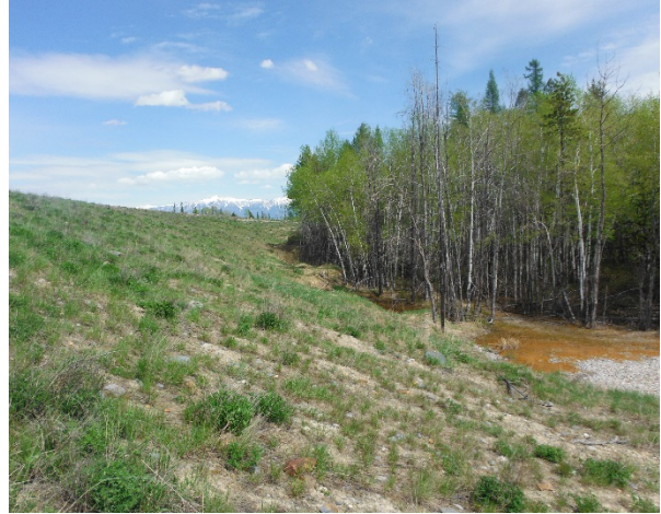
1.02: May 10, 2017 Seepage collecting at toe of dike.
