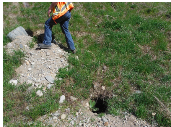
5.18: May 10, 2017 Large rodent burrows at toe of East Gypsum Dike
